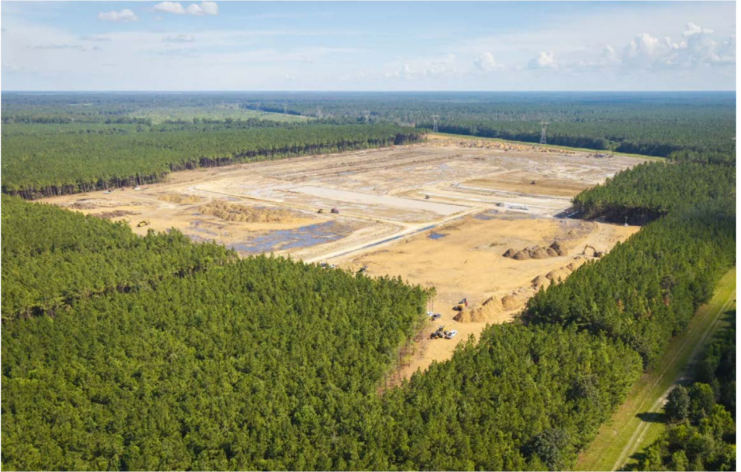
The site of an Entergy power substation photographed in Ouachita Parish, La., Tuesday, Sept. 1, 2026. (Staff photo by Sophia Germer, The Times-Picayune) STAFF PHOTO BY SOPHIA GERMER
